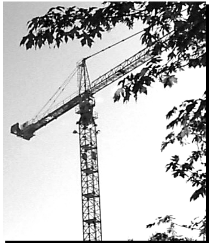
Tower crane sightings have been relatively rare over the last few years in western Canada. This one, framed by fall foliage, was spotted in Vancouver recently. Thanks to Don Bonokoski at the BC Construction Industry H & S Council for sending us this digital image over the net.
